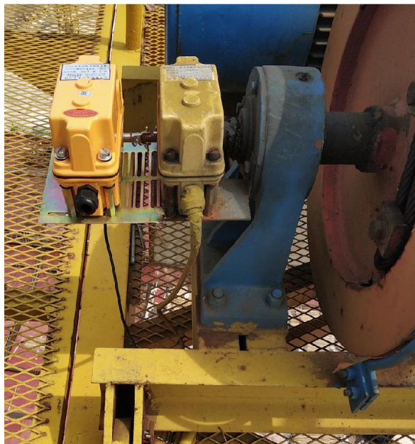
传感器加装在原来的限位器边上 Sensors install near the original limiters
